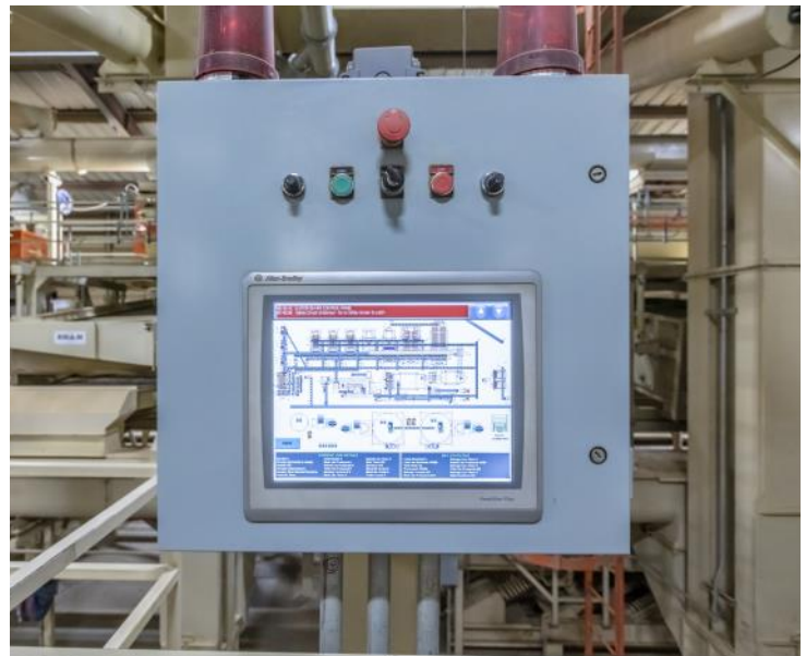
The new PLC in Kerman Plant #3.
